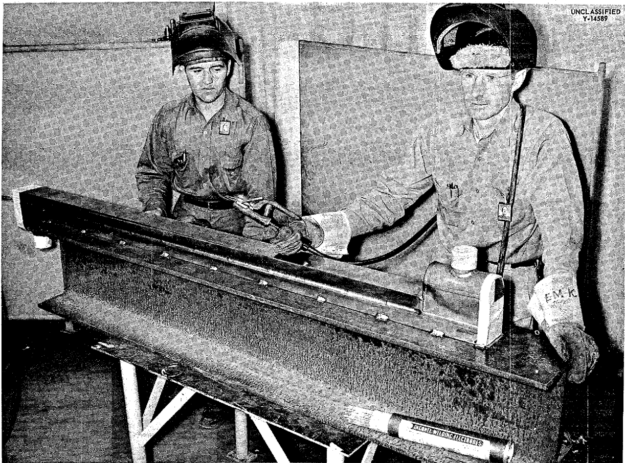
Fig. 6.14. Intermediate Heat Exchanger No. 2 After Completion of the Root Pass of the Pressure Shell Weld. Strongback used to minimize distortion.
