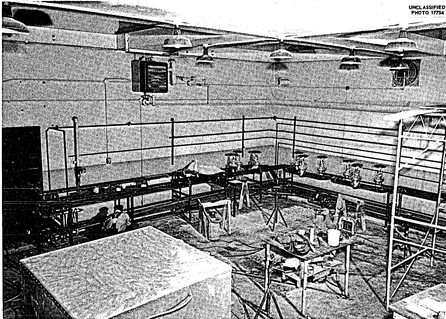
Fig. 1.5.13. View Showing the Southwest Corner of the Auxiliary Equipment Room. This room, which was used during ARE operation as the heat exchanger pit, is being modified to serve as the auxiliary equipment room and will house the lubricating oil pumping system and the hydraulic drive equipment.
