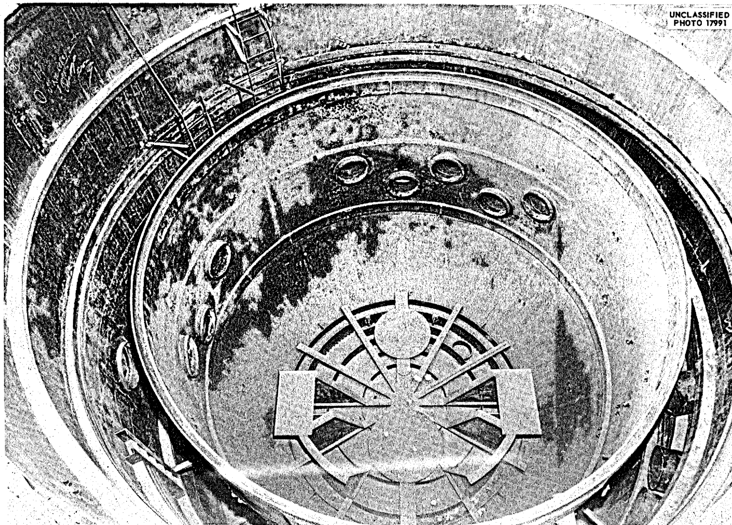
Fig. 1.5.4. View Looking North Across the Opened 7503 Cell Tank. The rectangular plates shown on the floor structure of the inner vessel will support the reactor. The circular plates shown will support the shielded fuel fill-and-drain tank and fuel removal tank. The 24-in.-dia nozzles through the side wall of the vessel will provide for the penetration of the instrumentation and control lines, lube oil lines, hydraulic drive lines, cooling water lines, gas lines, and heater leads to the cell equipment.
