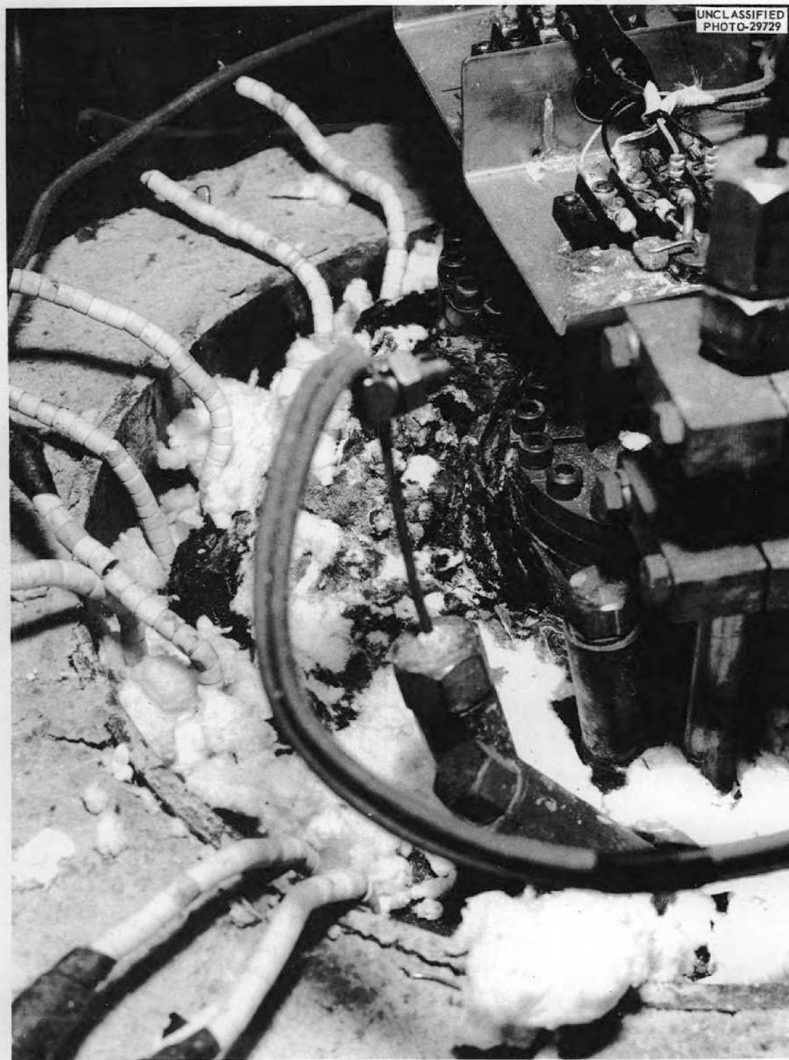
Fig. 1.3.13. A Pot of a Level-Element Testing Rig Showing Oxide Deposits Resulting from a NaK Leak.
