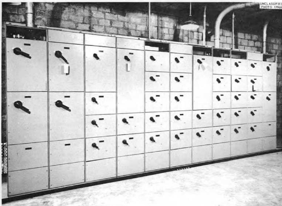
Fig. 1.1.17. A Section of the Motor Control Center. June 1956.
