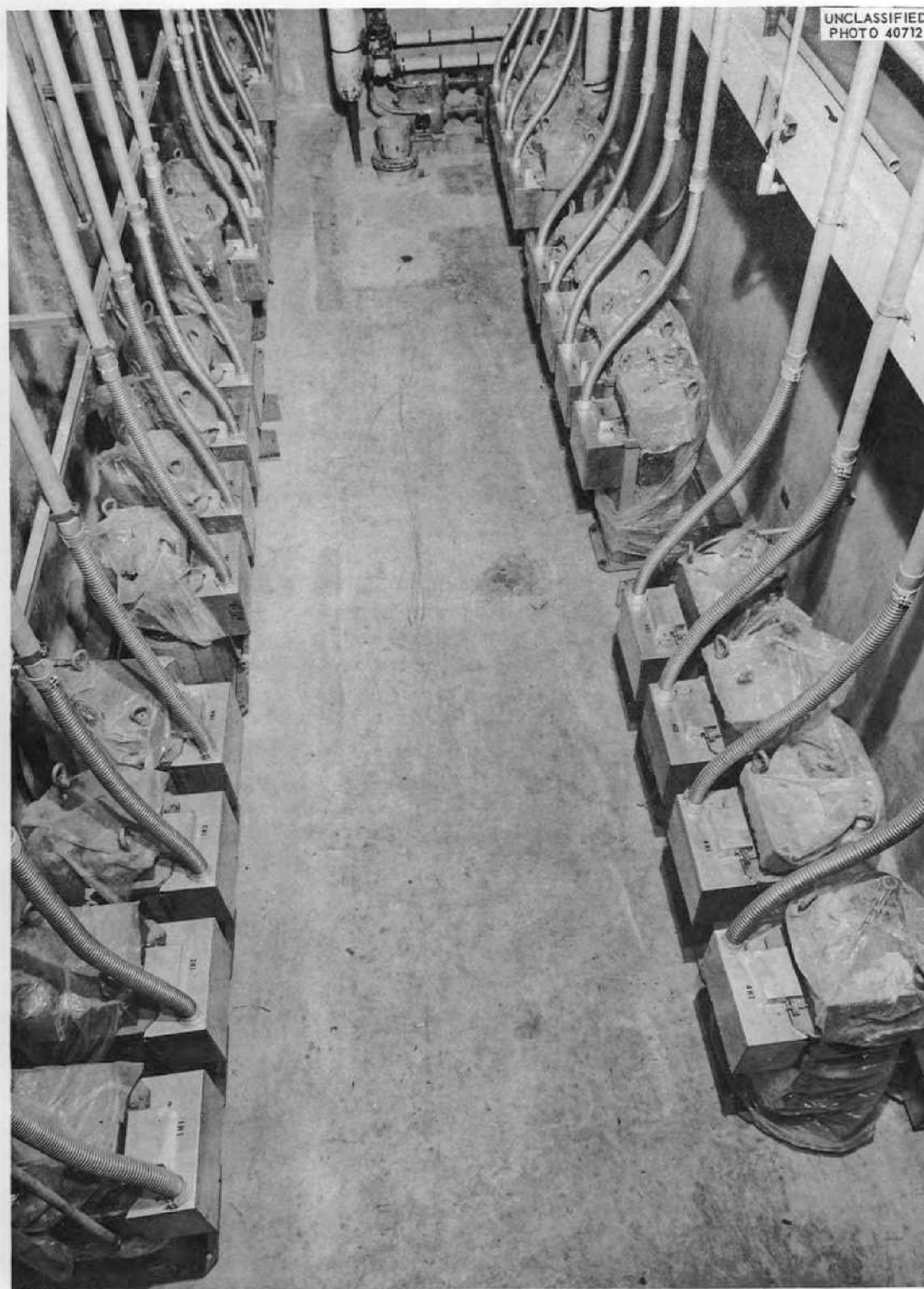
Fig. 1.1.21. Remotely Controlled Induction Voltage Regulators. April 1957.
