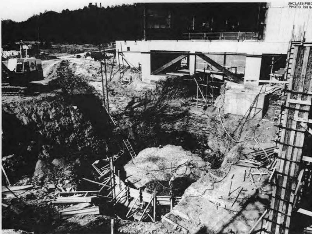
Fig. 3. View of Excavation, Showing the Highly Compacted Crushed Stone Subbase for the Cell Foundation.
