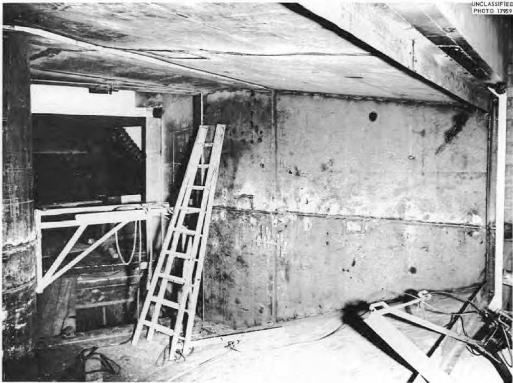
Fig. 5. View into the Main Air Duct from the West. In the background can be seen the guide vanes which are located at the base of the stack.
