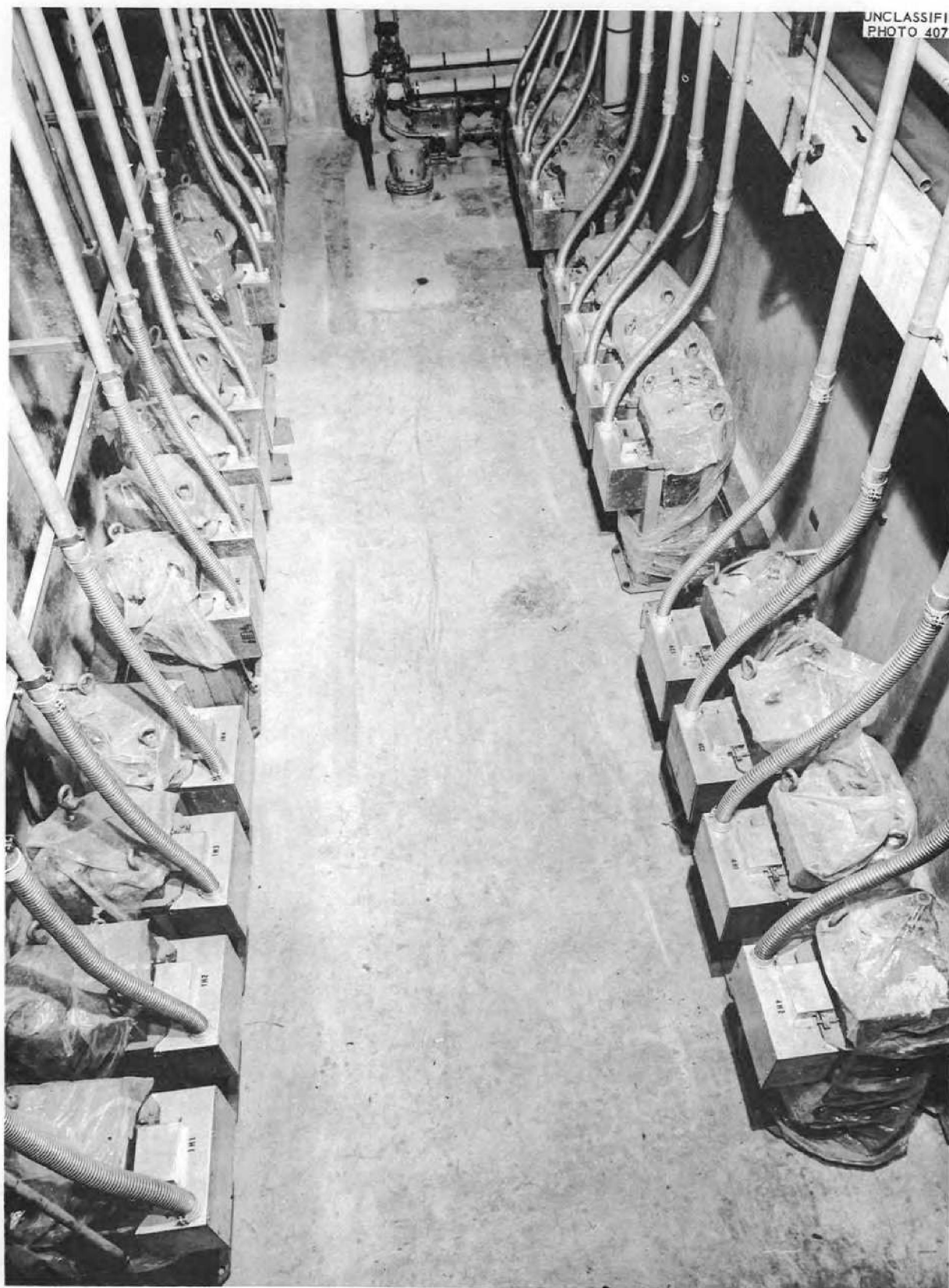
Fig. 14. The Regulator Pit in the North Basement. Some of the induction voltage regulators are shown.
