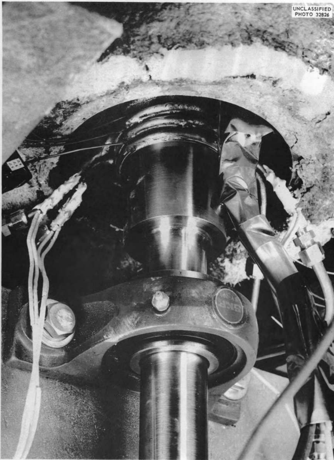
Fig. 1.2.4. Sealing Gland, Shaft, Cooling Coils and Thermocouples for Frozen-Lead Seal Test.
