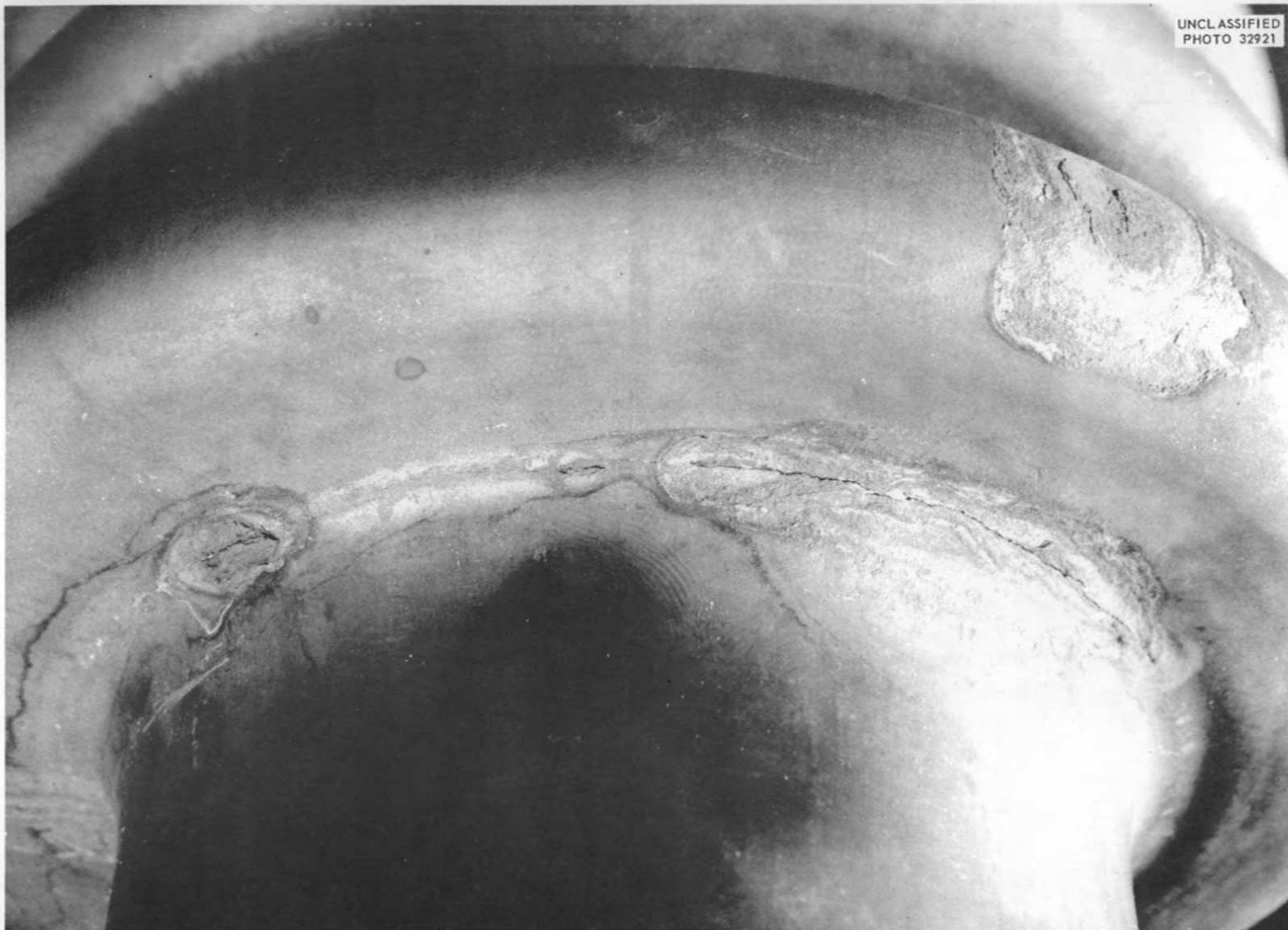
Fig. 1.2.10. Cracked Area of Flexonics Corp. Inconel Expansion Joint Bellows That Was Tested in a Molten Salt at 1300°F.
