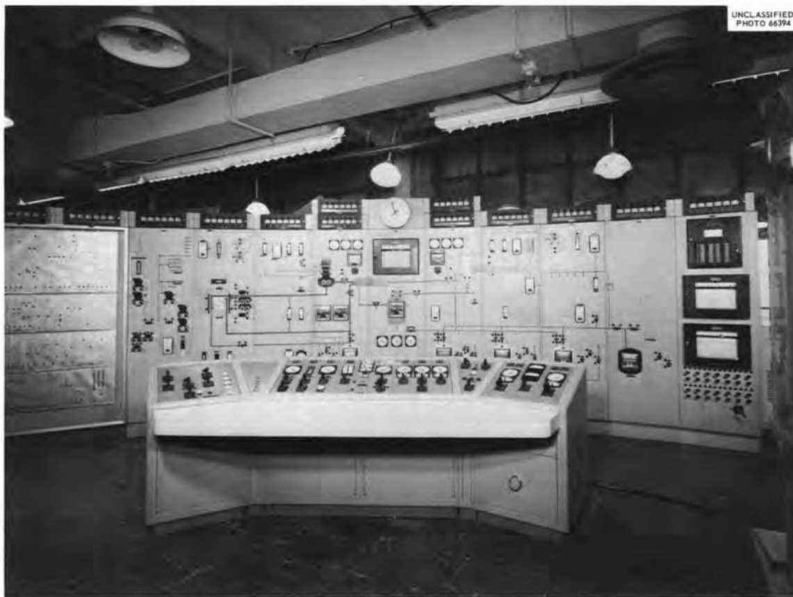
Fig. 10. MSRE Main Control Room.
