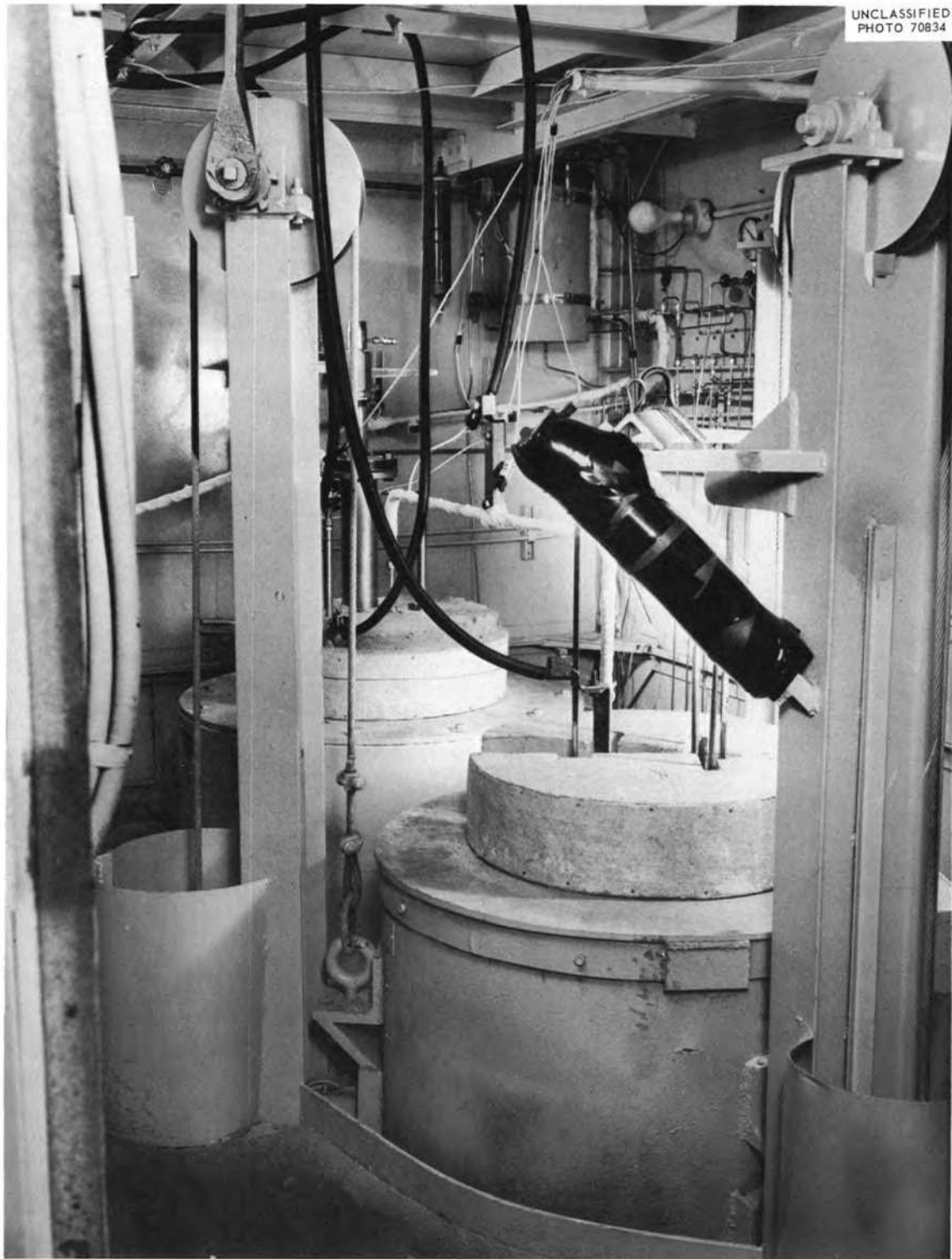
Fig. 5. Fluoride Production Facility - Batch Processing Unit.
