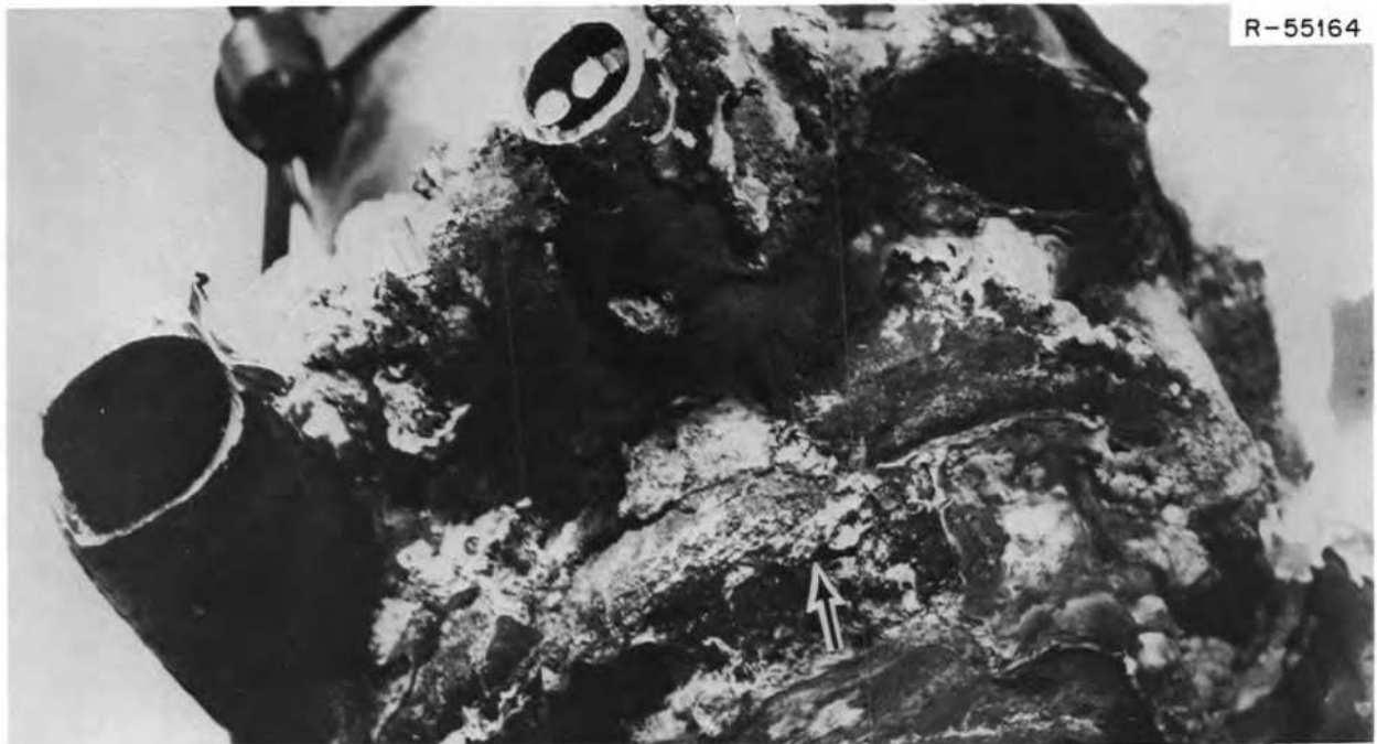
Fig. 13.31. Closeup of the bottom of freeze valve 105 showing the two gas outlet lines and one inlet line of type 304 stainless steel that was corroded completely. The crusty substance is the salt. Note that there is no salt in the air annulus.
