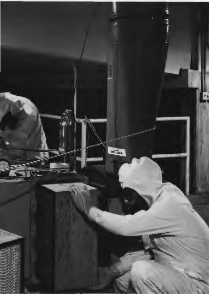
Maintenance of exhaust system in attic over Metals & Ceramics Division in 4500S.
